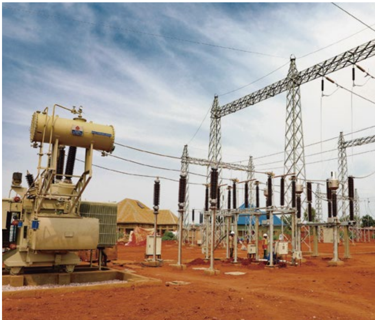
Our TFM operation completed an electrification project in the town of Tenke, demonstrating its commitment to addressing community development priorities and long-term infrastructure needs.
